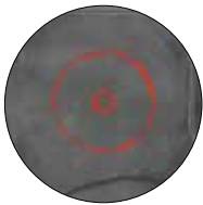
Plugged Sprinkler Running Sprinkler
